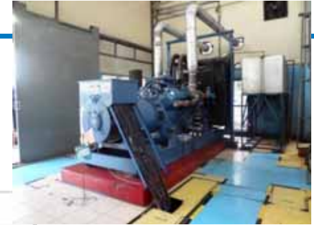
PLN diesel power plant
