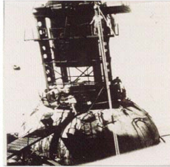
George Claude vertically fabricating and installing iron OTEC pipe off Brazil in 1930's.
