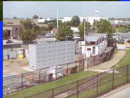
Three 600-HP compressors + 1 MW NaS battery
