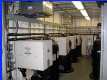
Containerized 7 Flywheel System
