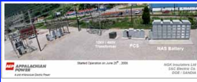
Charleston, WV Appalachian Power Substation
